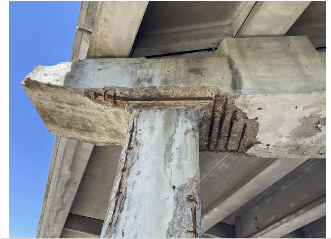
Bent 1, cap underside left end and under Bay A, serious spalling with exposed and debonded rebar
