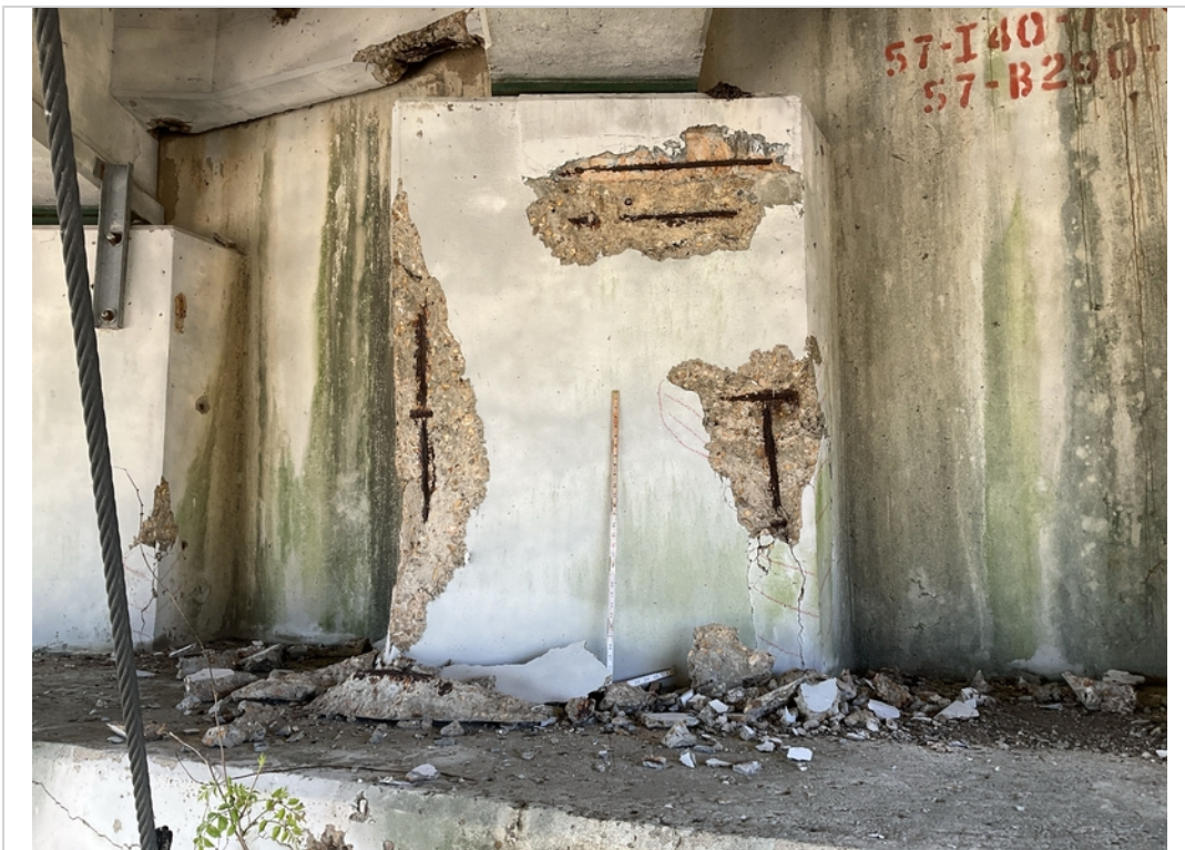
Abutment 1, pedestal B with spalling and exposed rebar throughout.
