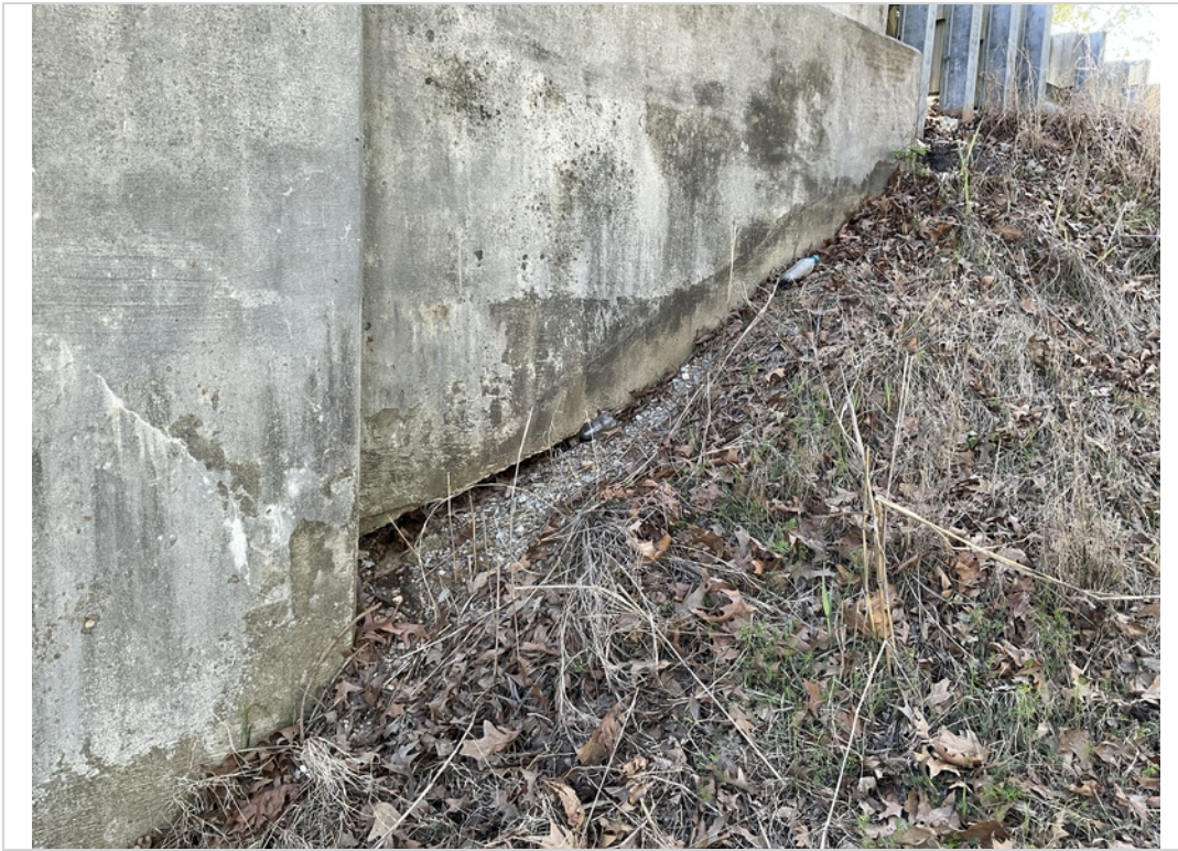
Abutment 2 right wing wall with undermining
