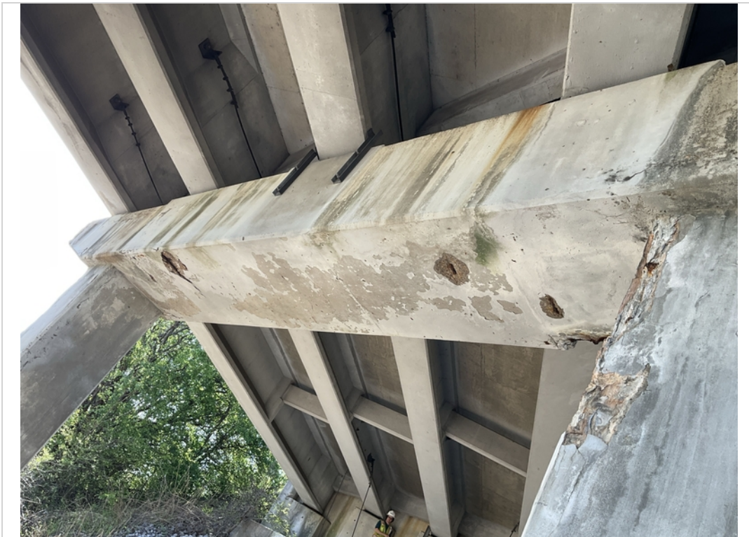
Bent 3 cap underside with multiple delaminated areas and spalls
