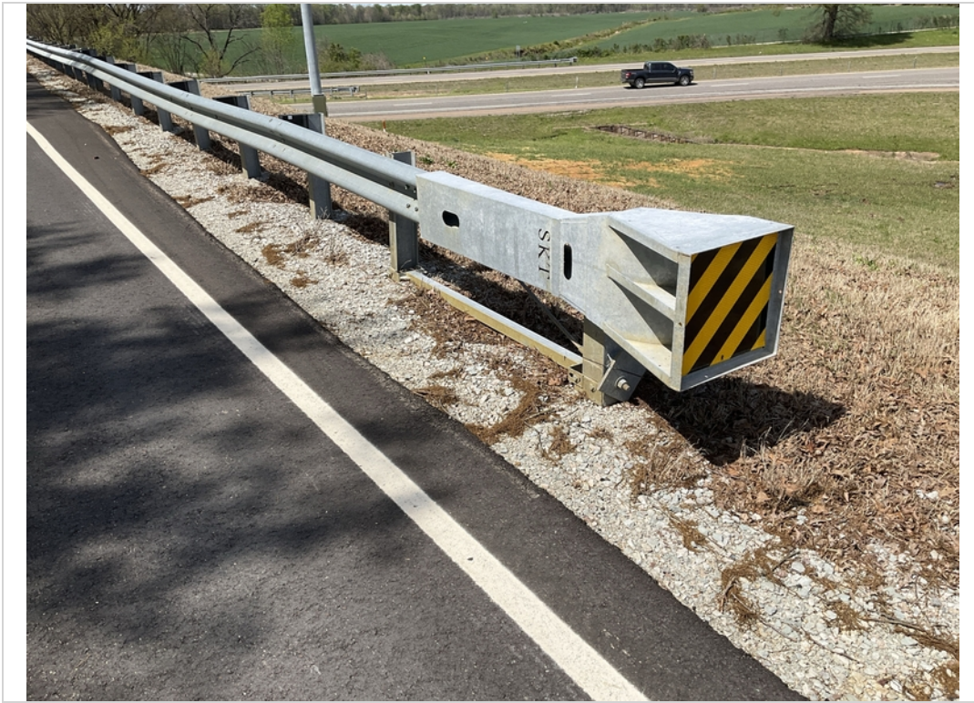
Approach 1 right termination (SKT impact attenuator)
