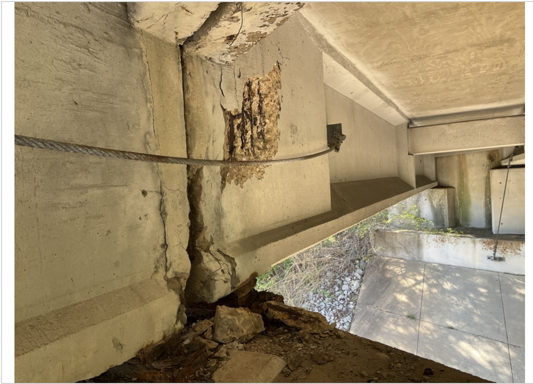
Beam A, over Bent 3, heavy spalling to web
