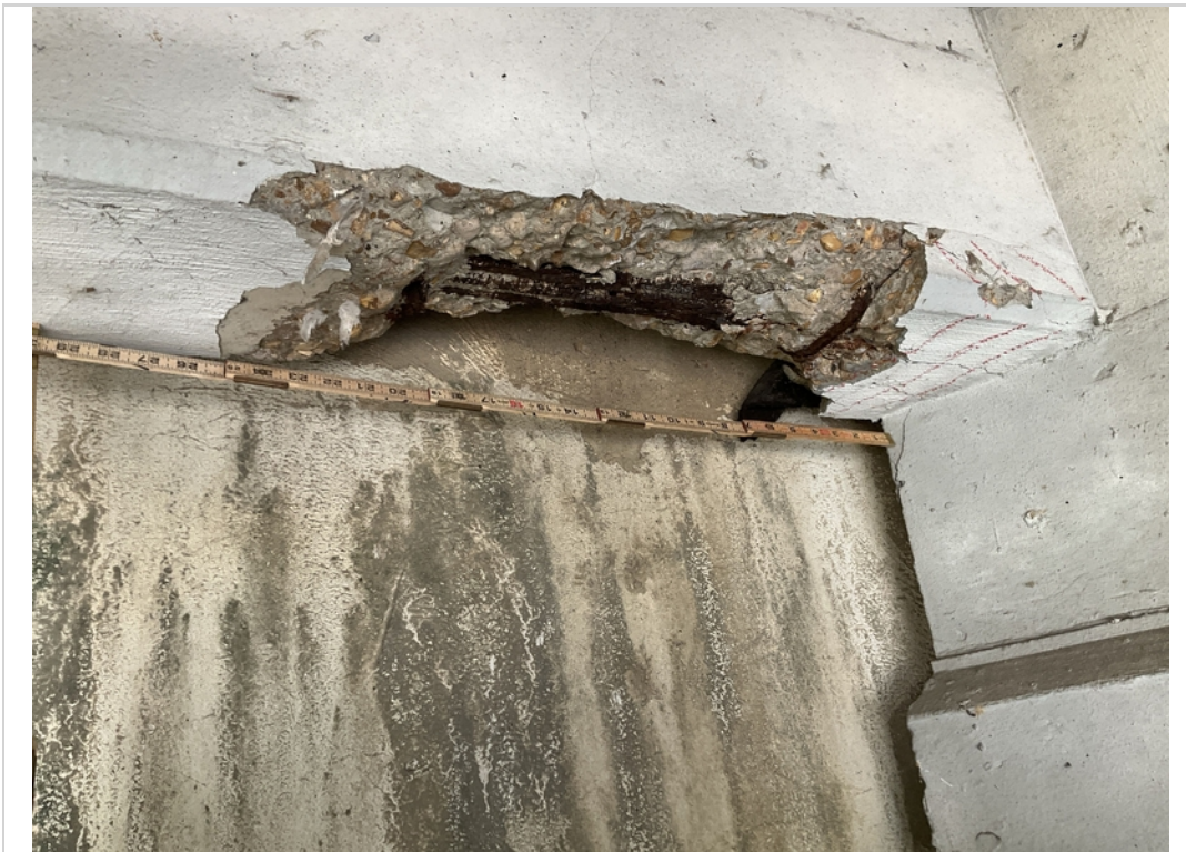
Span 1, End diaphragm Bay B at Beam B right side, Abutment 1, spall (26" x full width x 3" deep) with exposed corroded rebar.
