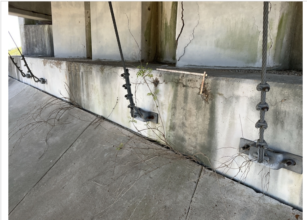
Abutment 1 cap with horizontal crack along top of cap (20' x 1/8" wide)
