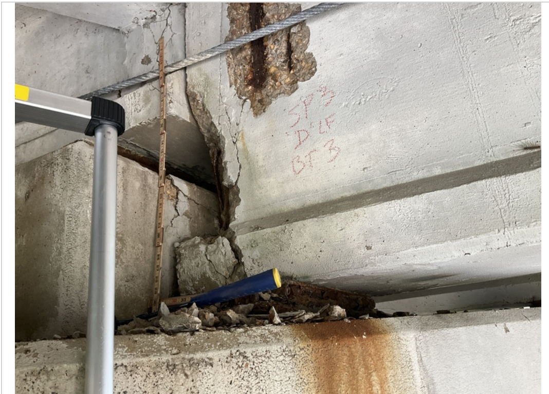
Beam D, Span 3, Bent 3, spalled beam end with exposed strand ends.
