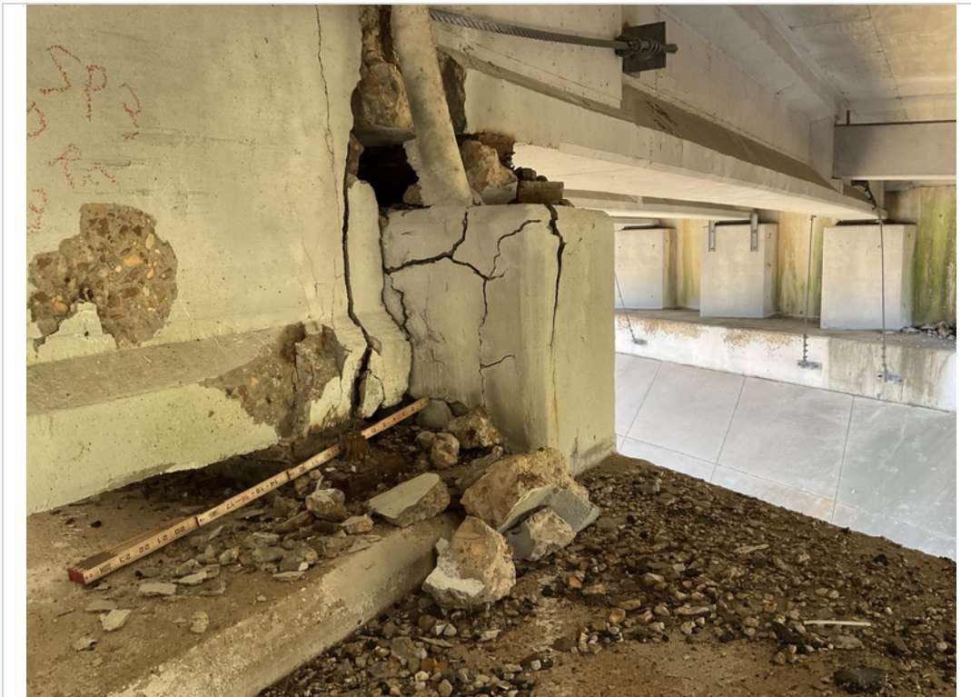
Beam D, Span 3, Bent 3, right face, beam end web spall with spalled and broken concrete and the beam end. Delaminated beam end, Span 4 pedestal with delaminated areas with wide cracking.
