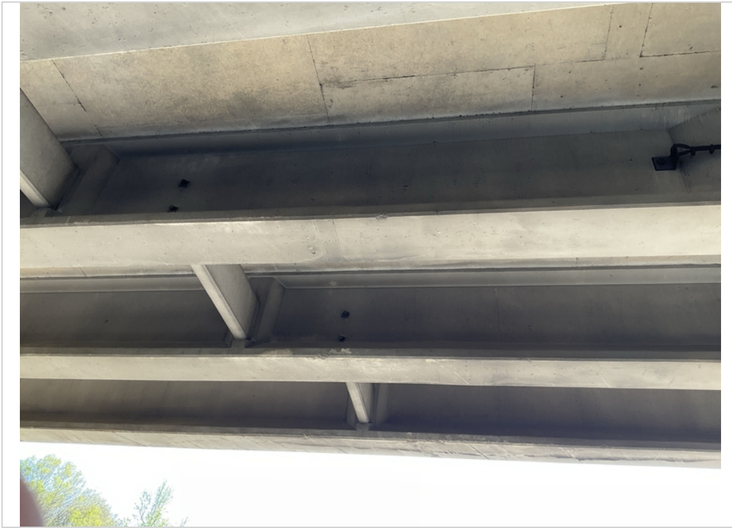
Beam C, Span 3, over right travel lane, minor bottom flange (right side) spall
