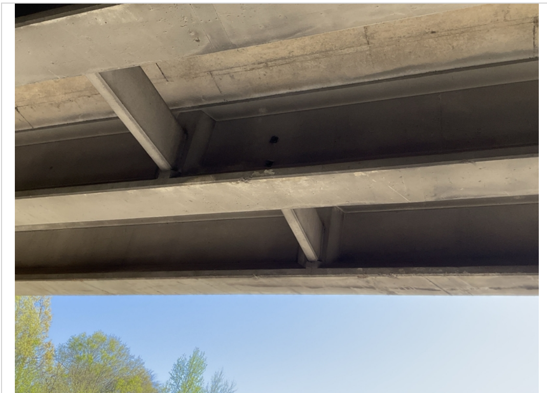
Beam B, Span 3, over right travel lane, minor bottom flange (right side) spall
