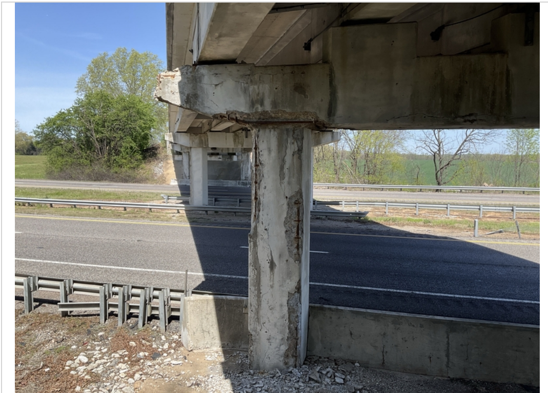
Bent 1, front face, left side cap and left overhang, widespread cracking with delaminated areas and spalls exposing rusted rebar
