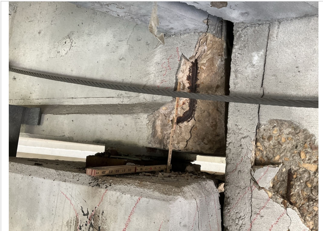
Beam C, Span 1, Bent 1, beam end spalls with exposed rebar and open cracking.
