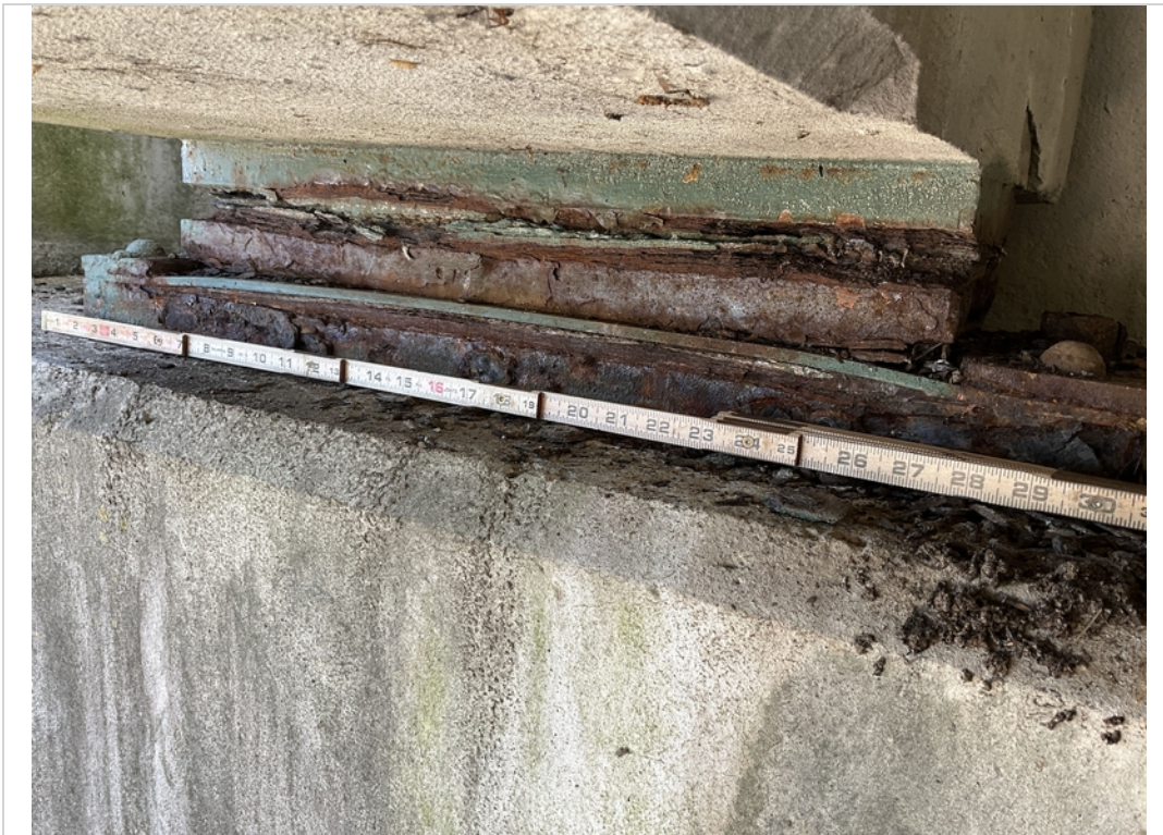
Abutment 1, Bearing E, severe corrosion with pack rust and section loss. Bearing is lifting due to pack rust.
