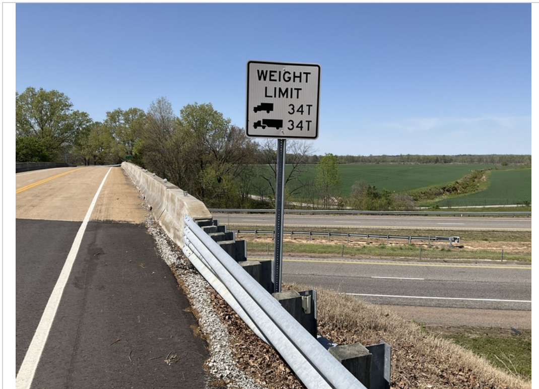
Approach 1, right corner, weight limit sign (34T restriction)
