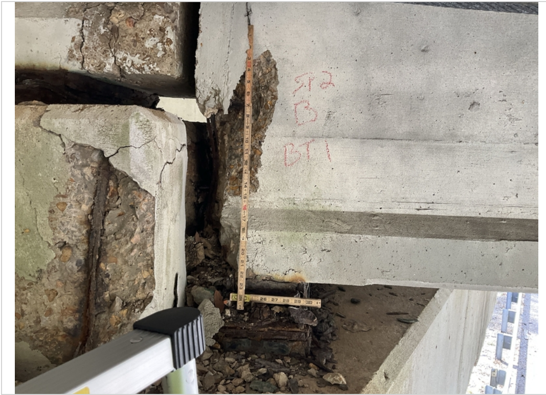
Beam B, Span 2, Bent 1, beam end spalls past bearing exposing stirrups and ends of P/S strands. Spalling with exposed and corroded rebar at the span 1 girder pedestal (left side of photo).
