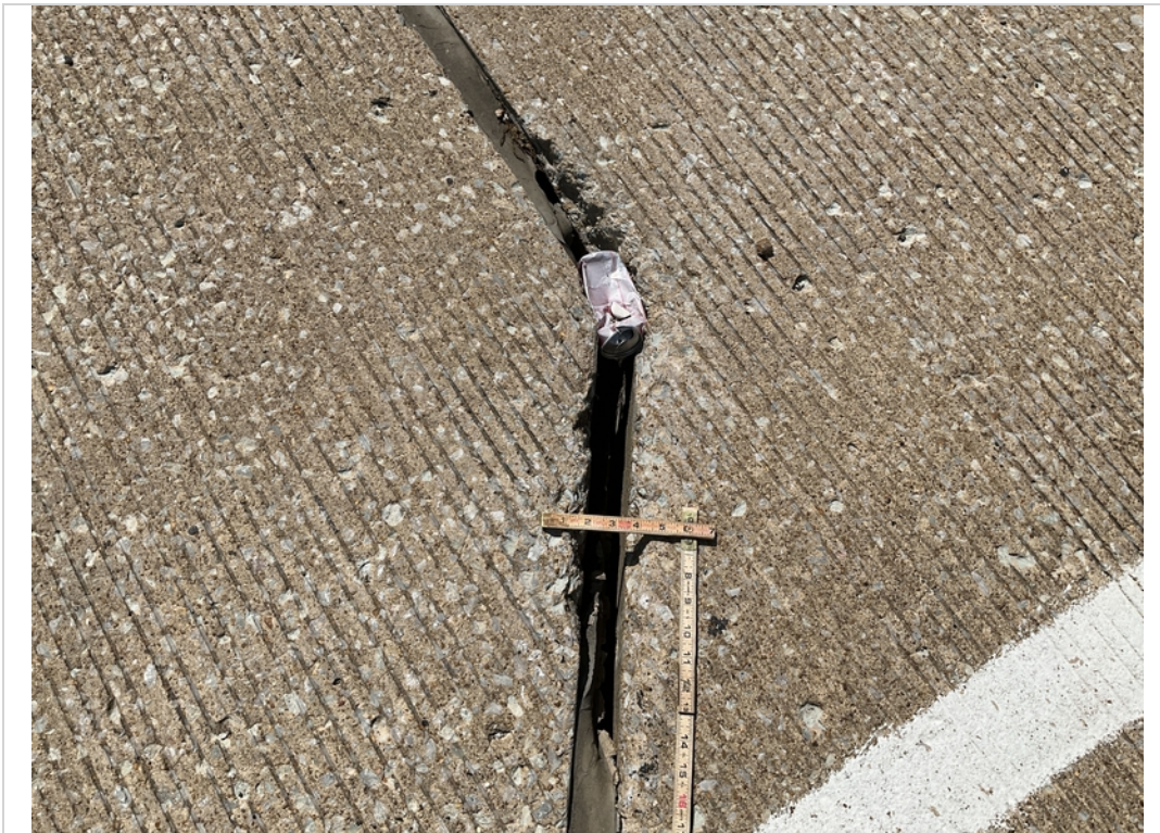
Joint over Bent 1 with sections of failed poured sealant allowing water to drain directly onto beam ends and substructure
