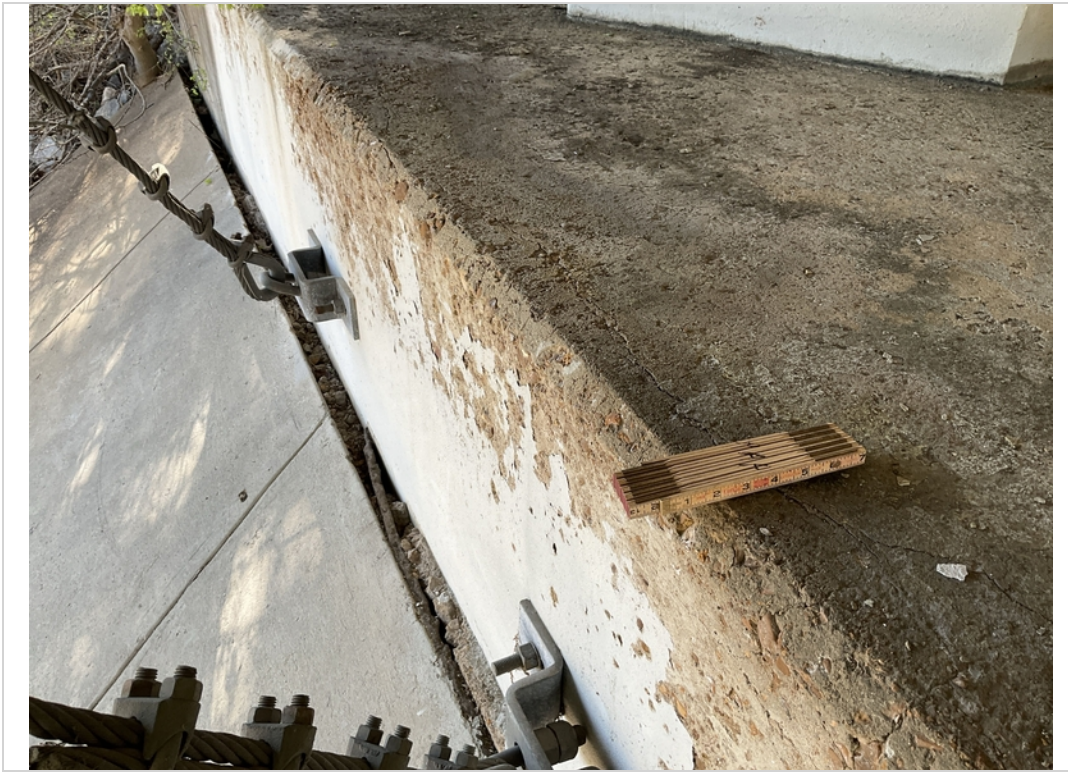
Abutment 2 cap with cracks in the top face adjacent to corner
