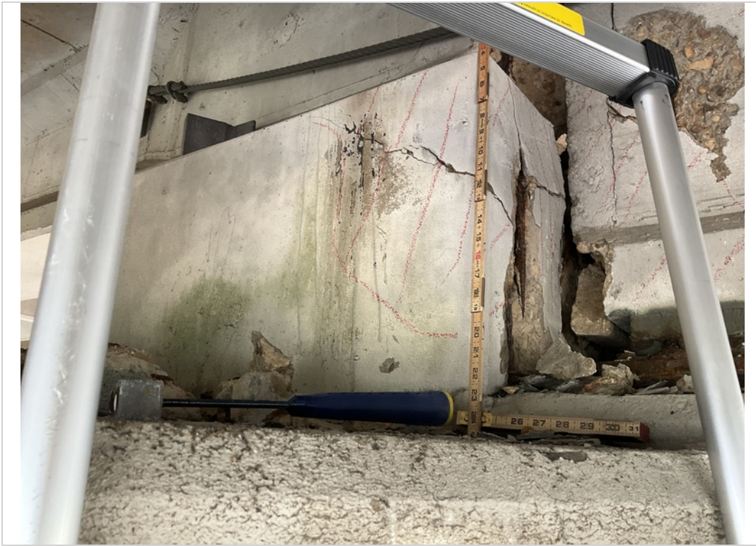
Pedestal for Beam C at Bent 1, delamination with adjacent spalling with exposed rebar.
