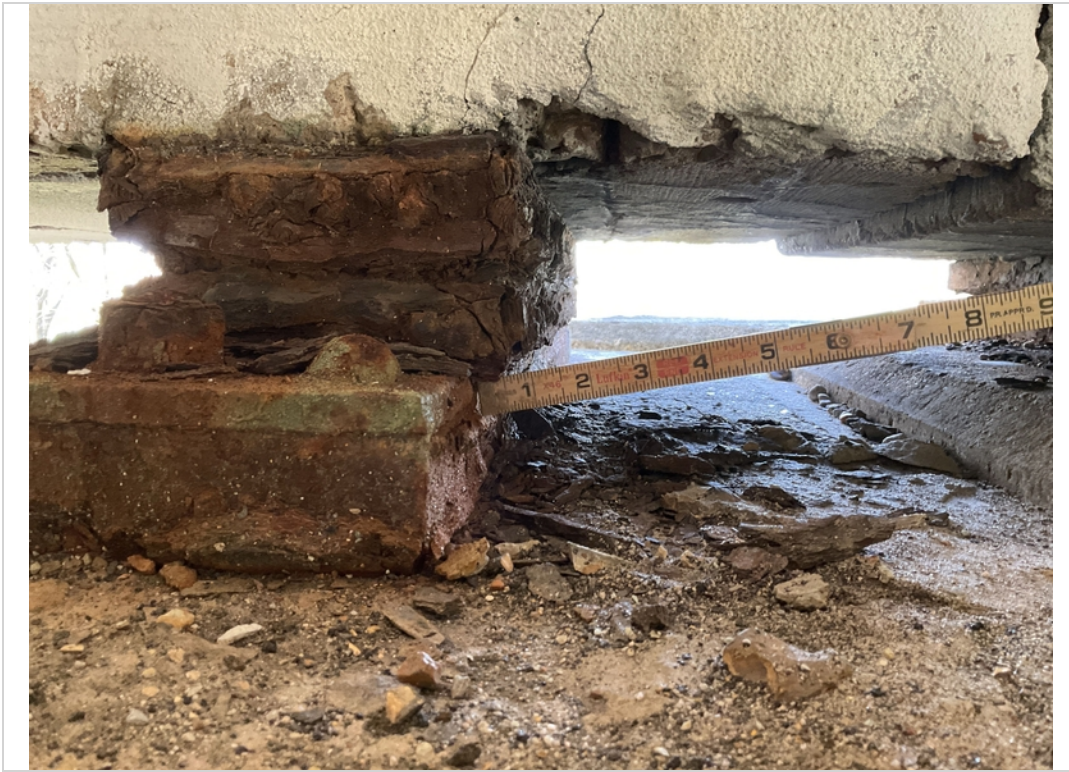
Bearing E, Span 4, Bent 3, over-expanded with major corrosion.
