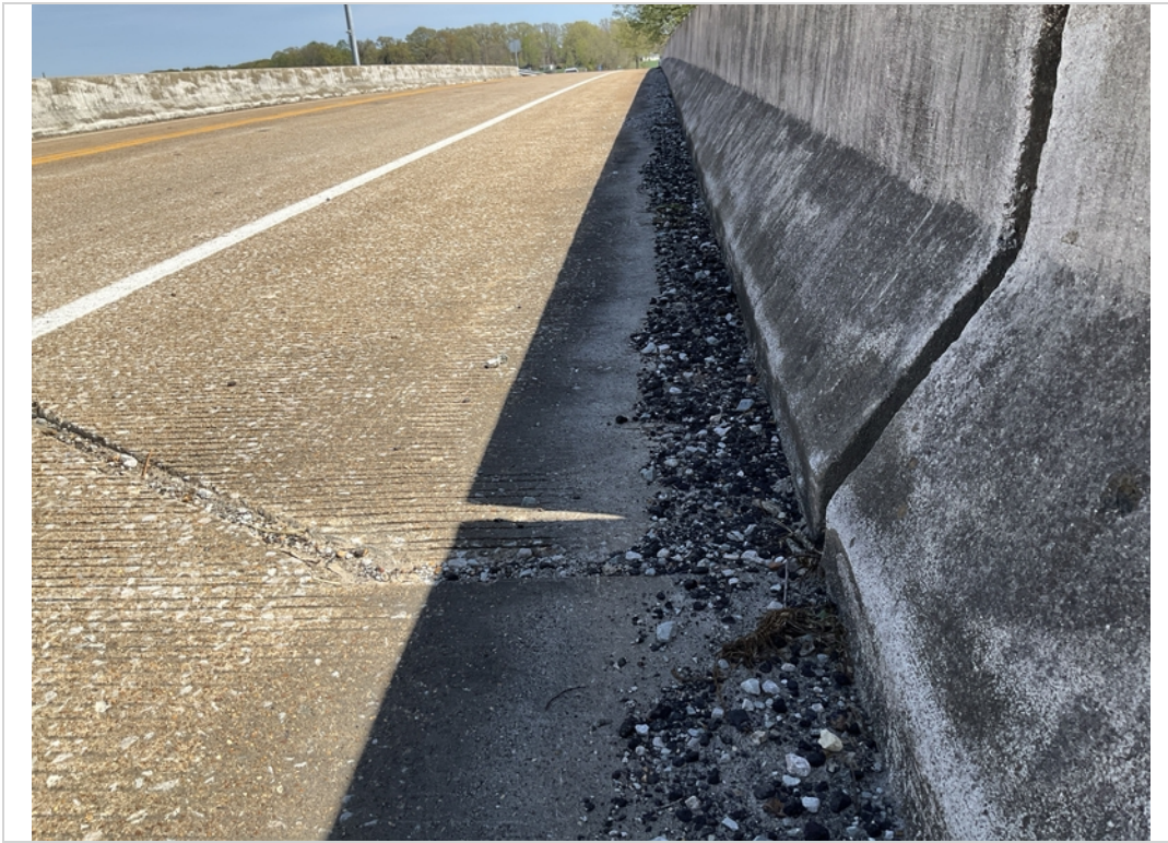
Left gutter line with minor debris
