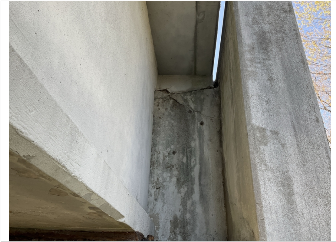
Abutment 2 backwall under right deck overhang, delamination with minor spall.
