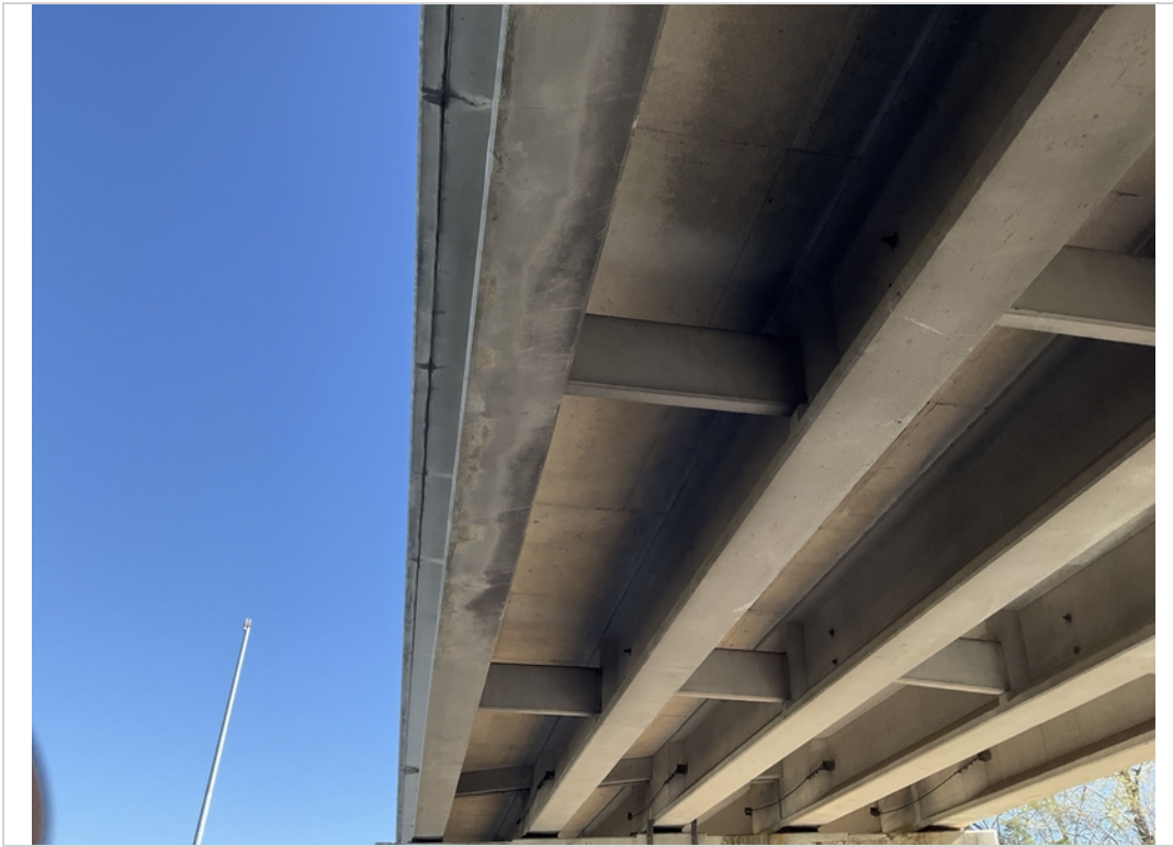
Beam E, Span 3, over right travel lane, surface scrapes on beam underside
