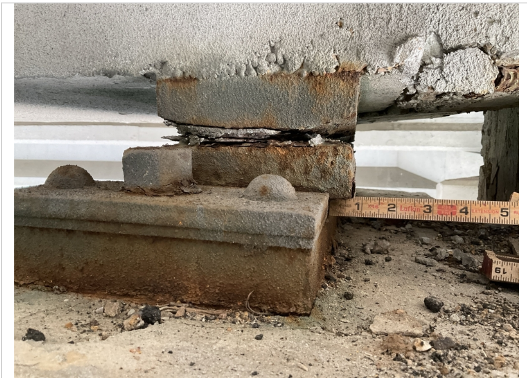
Bearing C, Span 4, Bent 3, over-expanded and heavily rusted with pack rust lifting the bearing
