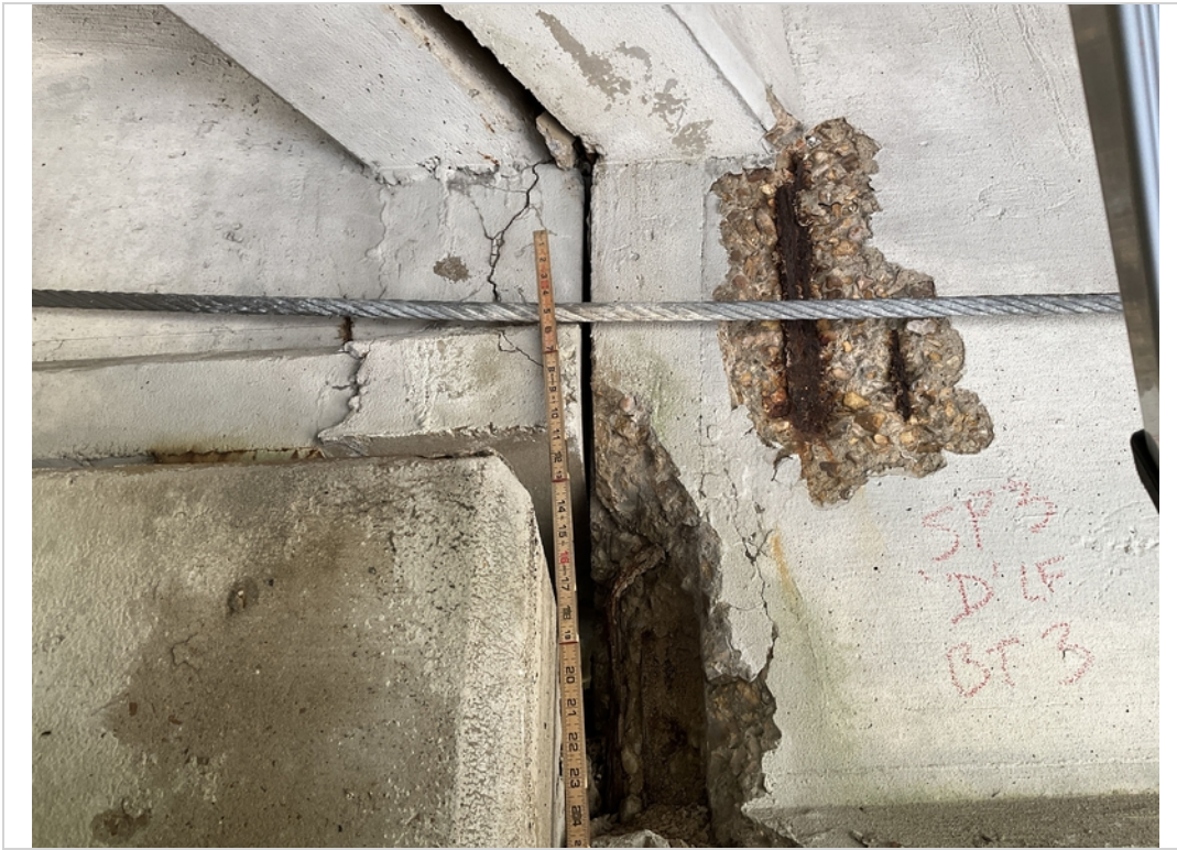
Beam D, Span 3, Bent 3, spalled beam end with exposed strand ends (right side of photo)
