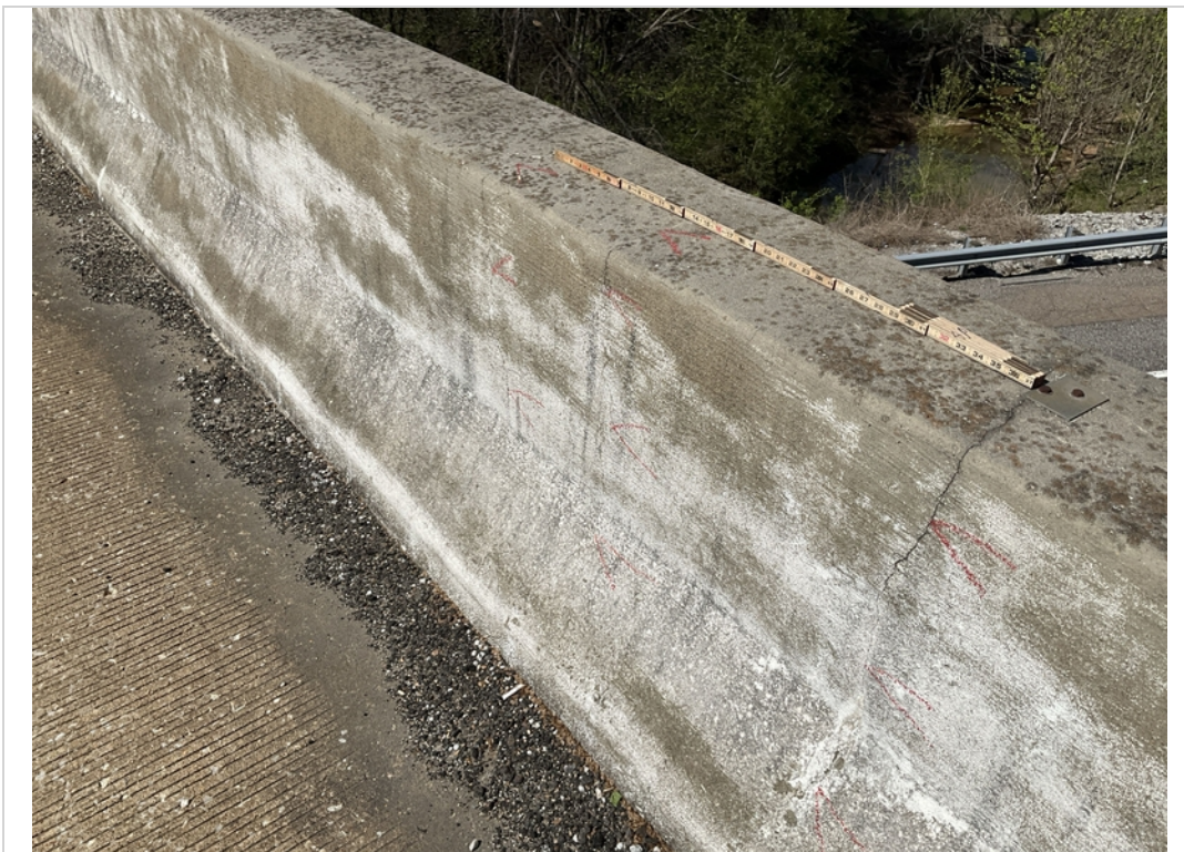
Right rail, span 3, vertical cracks (1/32" x full height), typical throughout all spans
