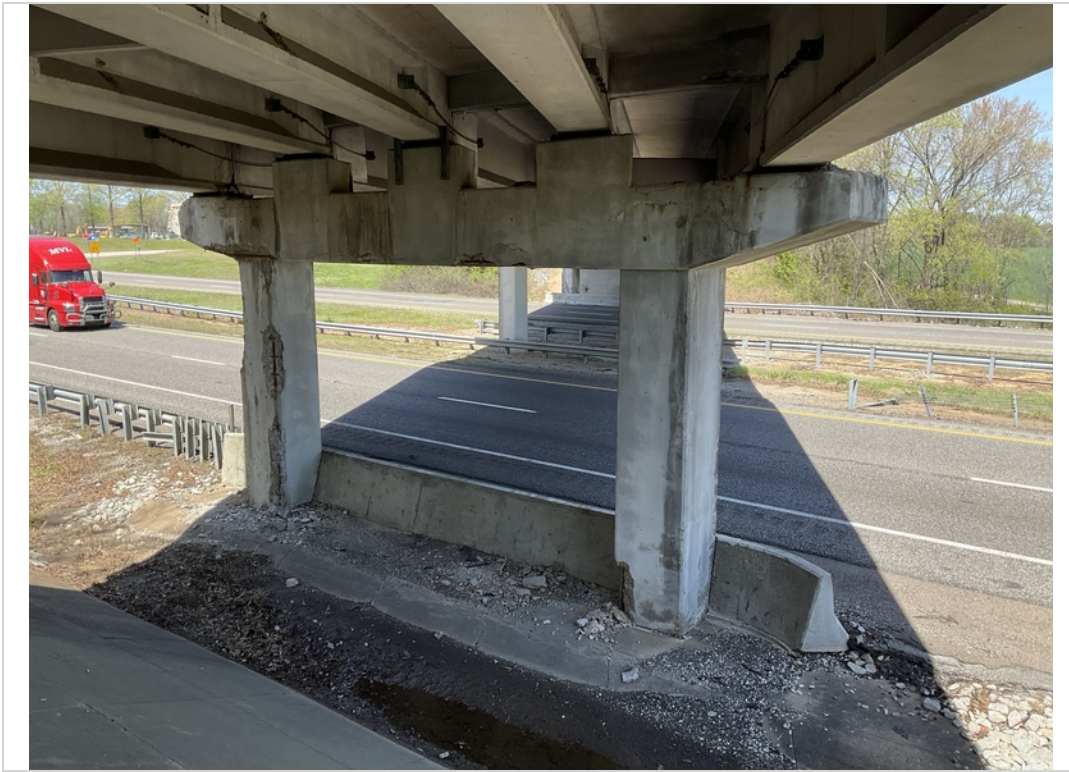
Bent 1, front face with significant spalling and delaminated areas throughout the columns and cap
