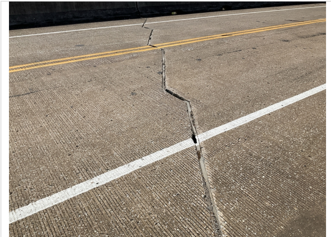
Joint over Bent 3 with failed sections of poured sealant allowing water to drain into the superstructure and substructure
