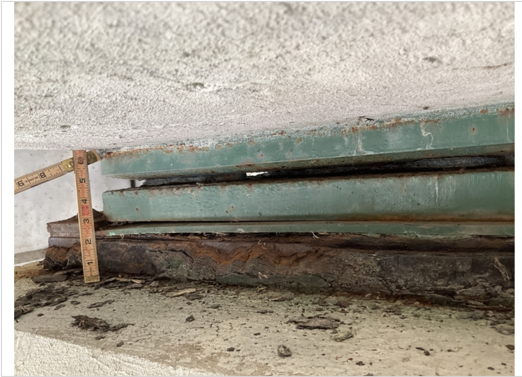
Abutment 1, Bearing D, pack rusting lifting the bearing and causing non-uniform bearing. Pack rust is 1/2" thick between sole plate and bearing plate with laminar rust along masonry plate. Missing anchor bolt at both sides.
