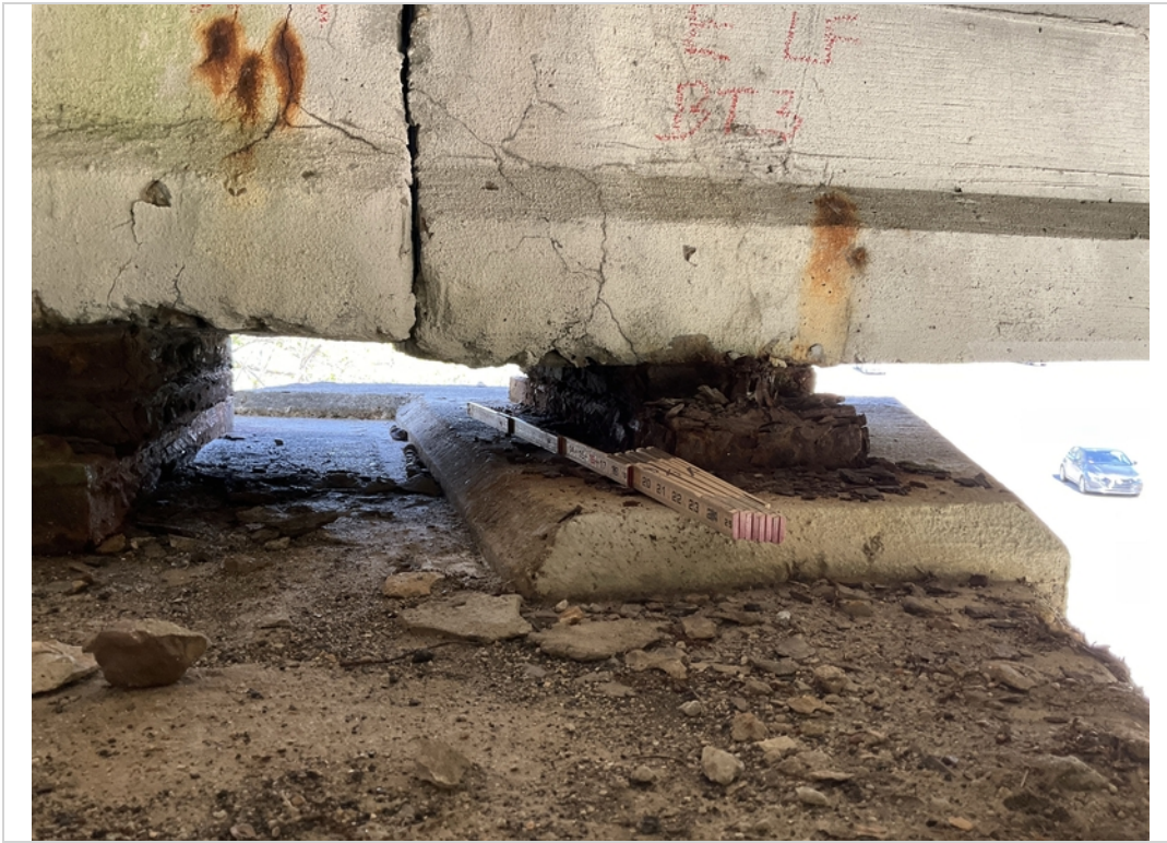
Bearing E, Span 3, Bent 3, typical corrosion with laminar rust and section loss
