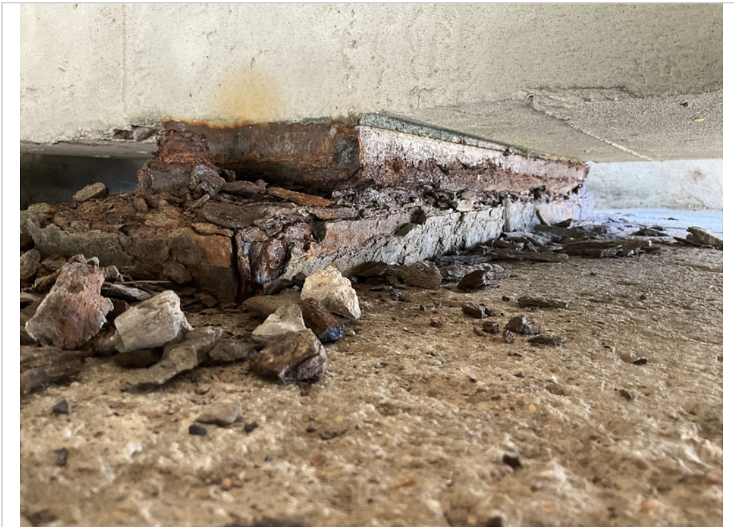
Bearing E at Abutment 2, Span 4, heavy corrosion with pack rust and section loss
