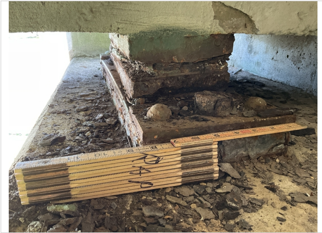
Abutment 1, Bearing E, severe corrosion with pack rust and section loss. Bearing is lifting due to pack rust.
