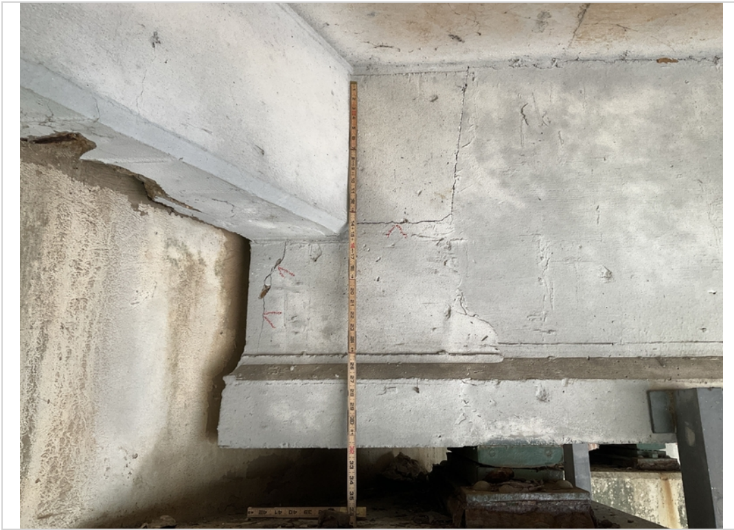
Span 1, Beam C, right side, abutment 1, minor beam end cracks with sound concrete adjacent to the end diaphragm
