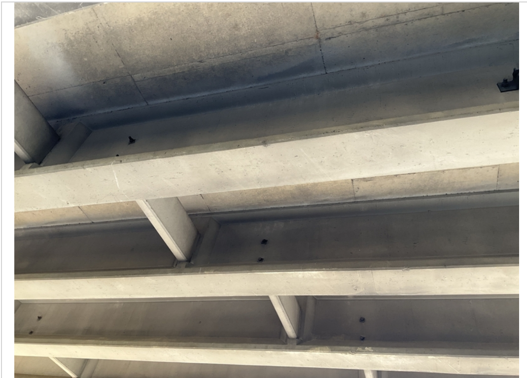
Beam D, Span 3, over right travel lane, minor bottom flange (right side) spall
