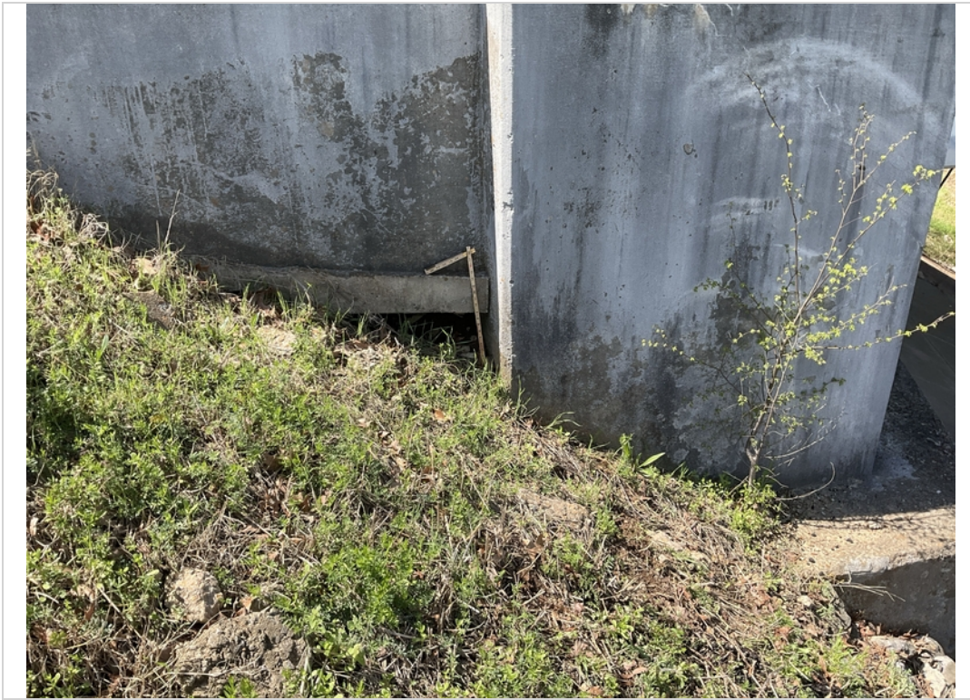
Abutment 1, right wing wall, localized undermining behind backwall
