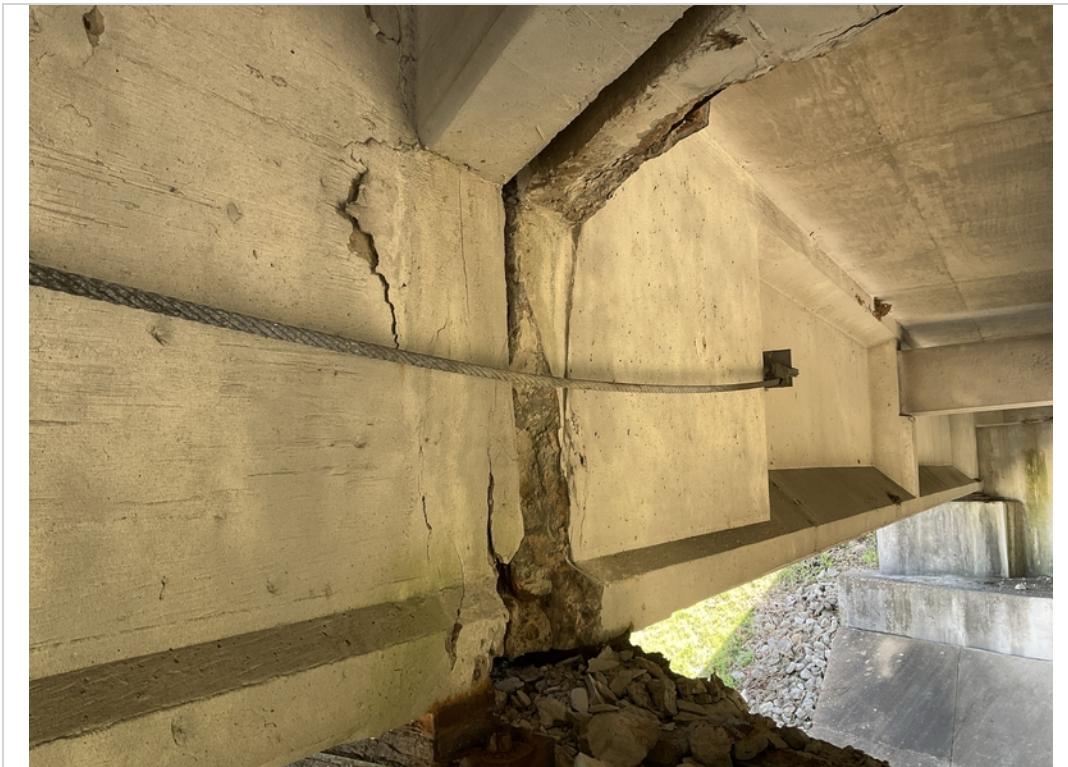
Beam E, Span 2 and 1 over Bent 1, typical beam end delamination and spalls.
