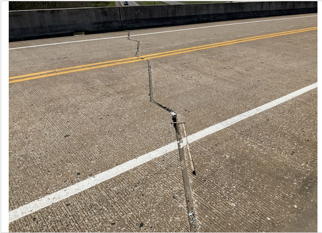
Joint over Bent 1 with sections of failed poured sealant allowing water to drain directly onto beam ends and substructure
