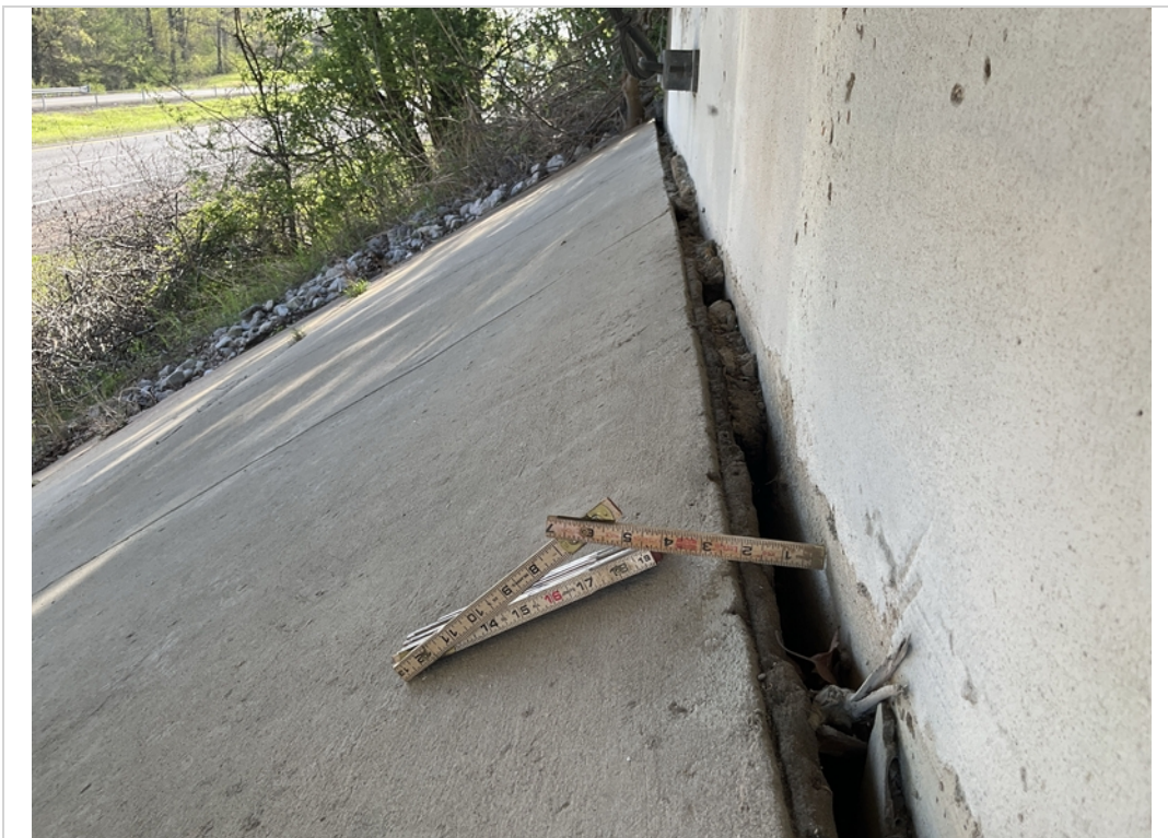
Abutment 2 slope protection pulling away from stem
