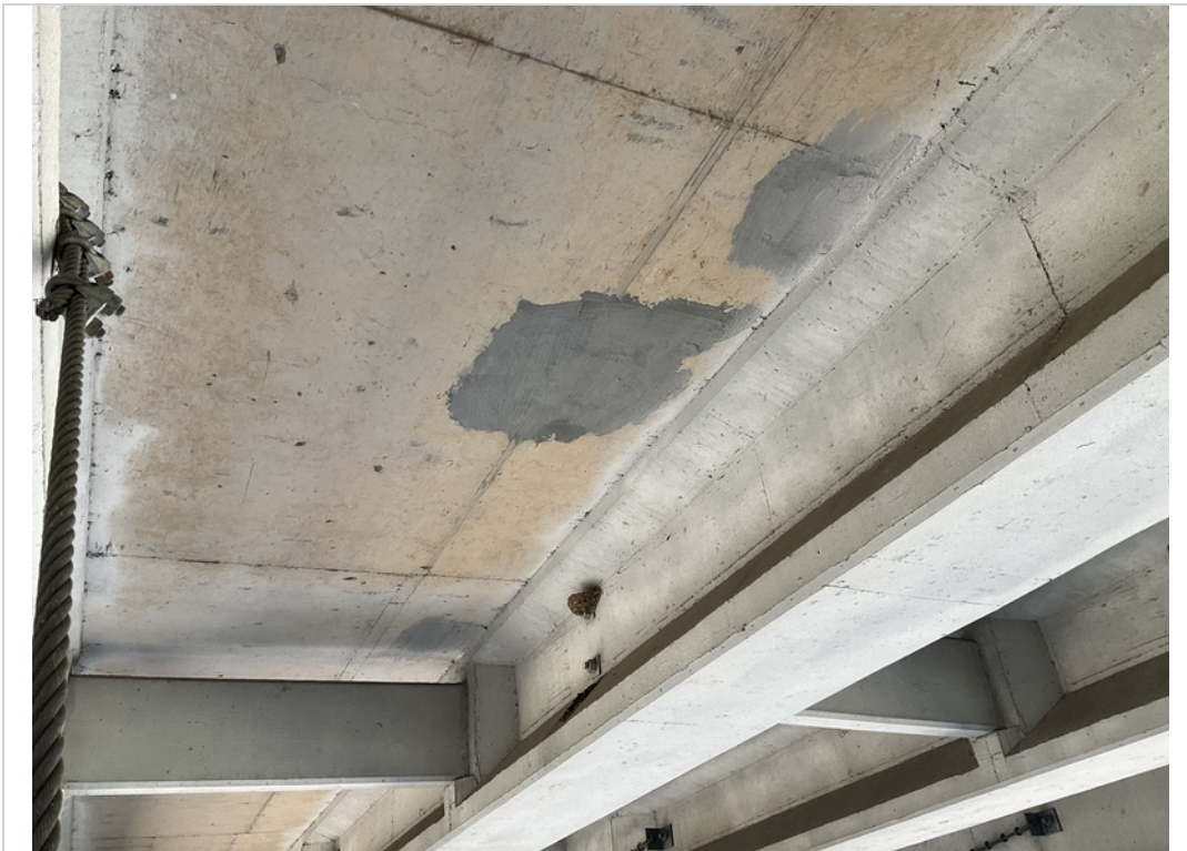
Span 1, deck underside, Bay B adjacent to Beam C, (3) patches (1'x1', 3'x3', 1'x1')
