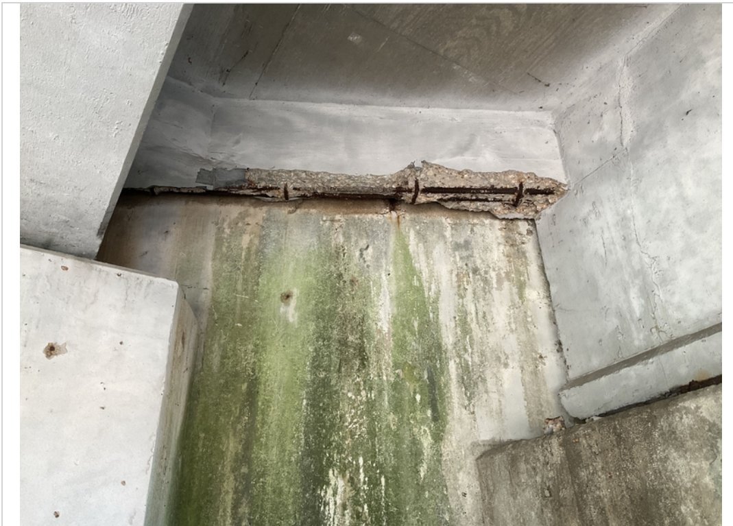
End diaphragm between Beams D/E at Abutment 2 with spalling throughout and exposed rebar with active corrosion
