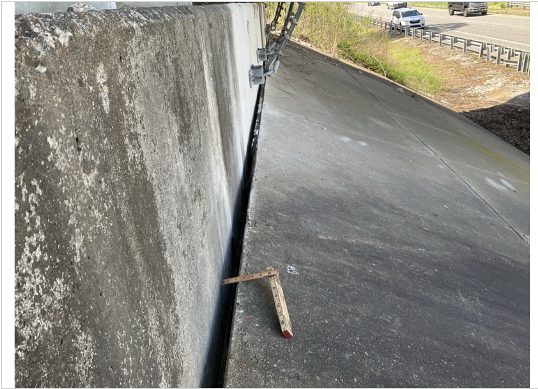
Abutment 1 slope protection looking left, separating from the stem face
