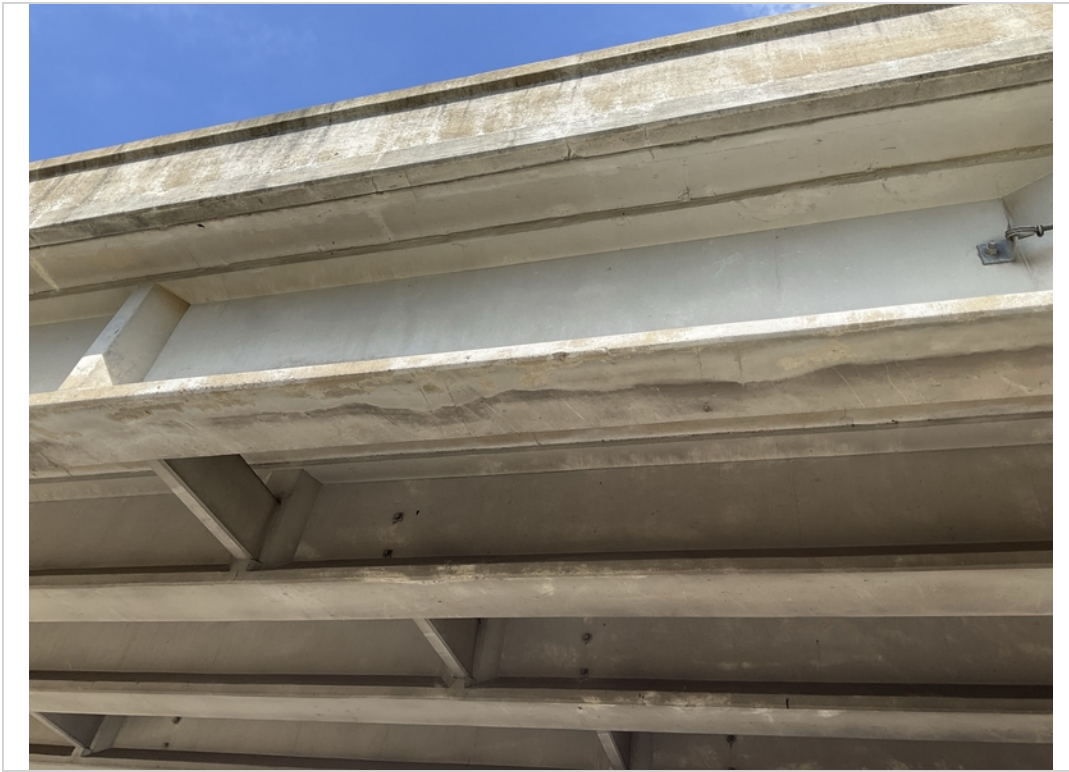
Beam A, Span 2, left corner over right travel lane, isolated minor impact spall on bottom flange corner with surface scrapes marks on underside
