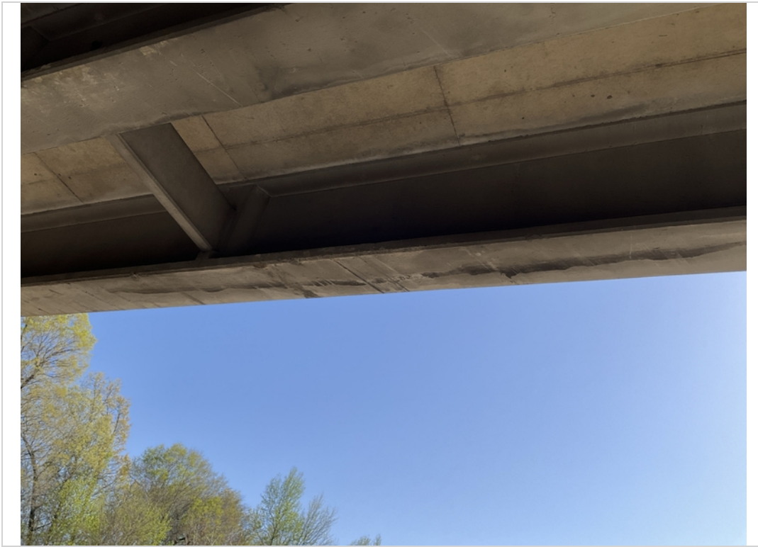
Beam A, Span 3, right bottom flange over right travel lane, impact spalls to bottom flange corner with multiple scrape marks (some appear to be up to 1/8" deep)
