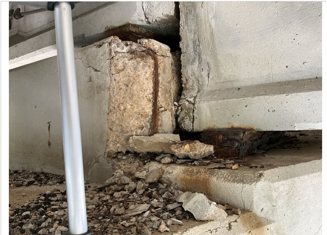
Pedestal for Beam B, Span 4, Bent 3, typical spall with exposed rebar
