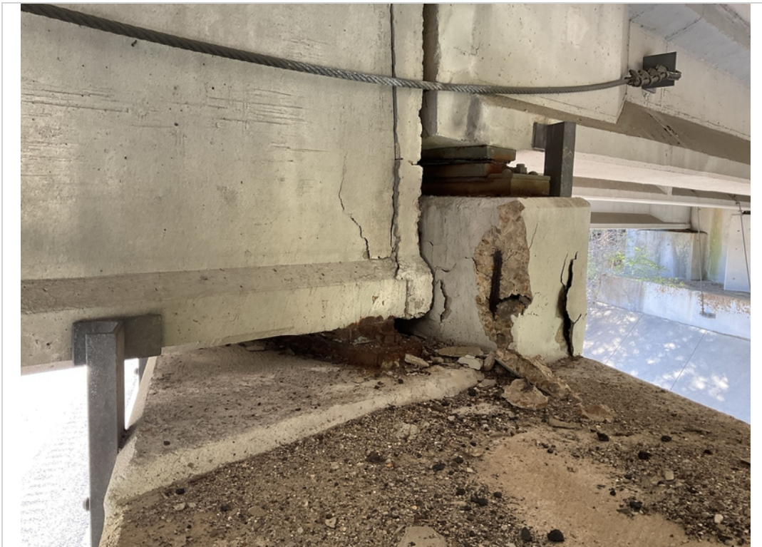
Beam C left face, Span 3 and 4 over Bent 3, spalling to the pedestal. Delaminated beam ends
