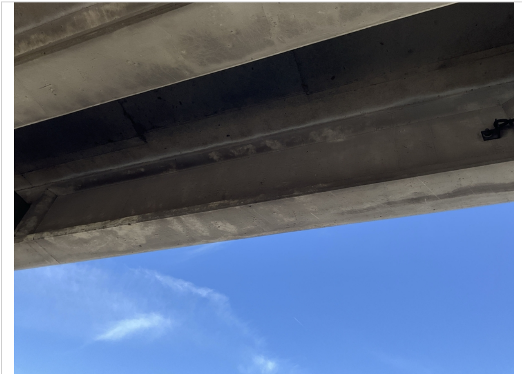
Beam E in Span 2, near Bent 1, minor surface scrapes on beam underside over right travel lane
