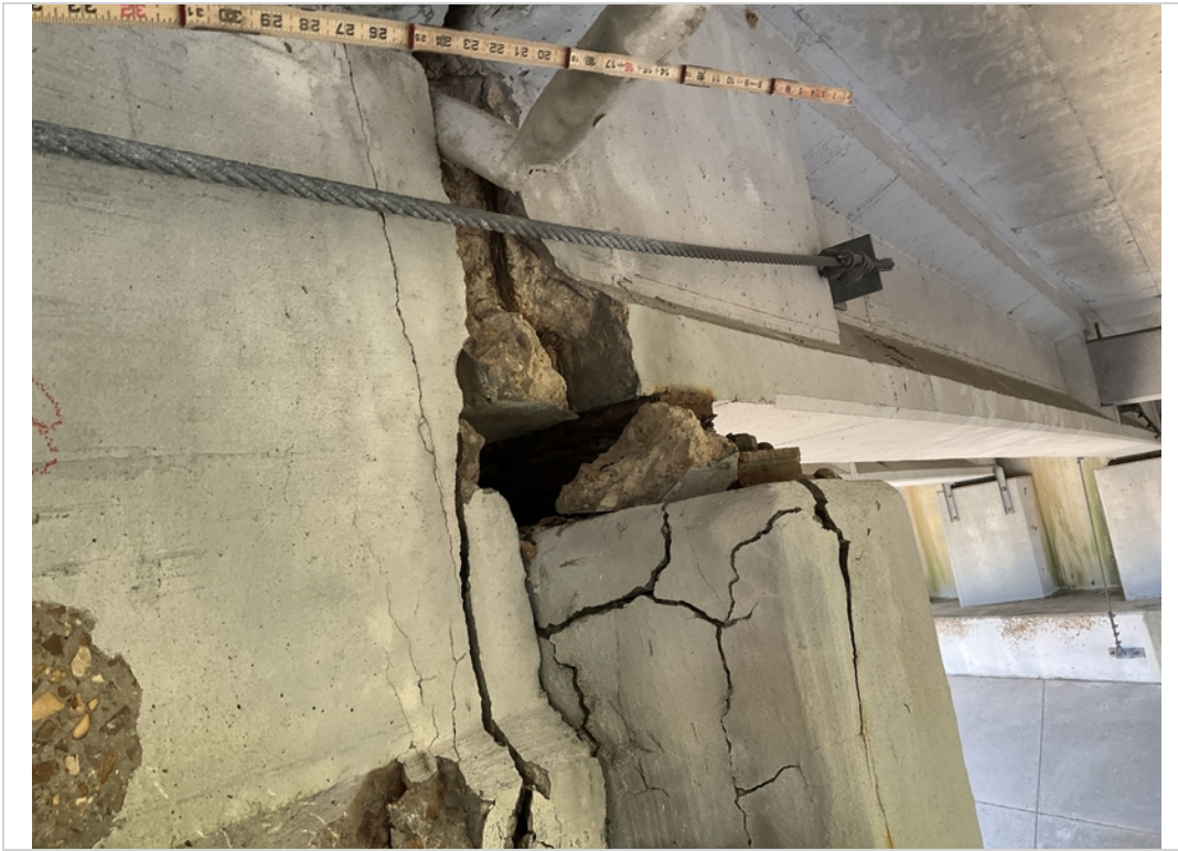
Beam D, Span 4, Bent 3, right face, beam end spall (right side of photo). Note the delaminated and heavily cracked pedestal.
