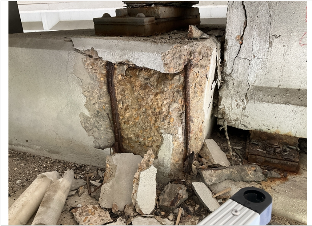
Pedestal for Beam C, Span 4, Bent 3, typical spall with exposed rebar
