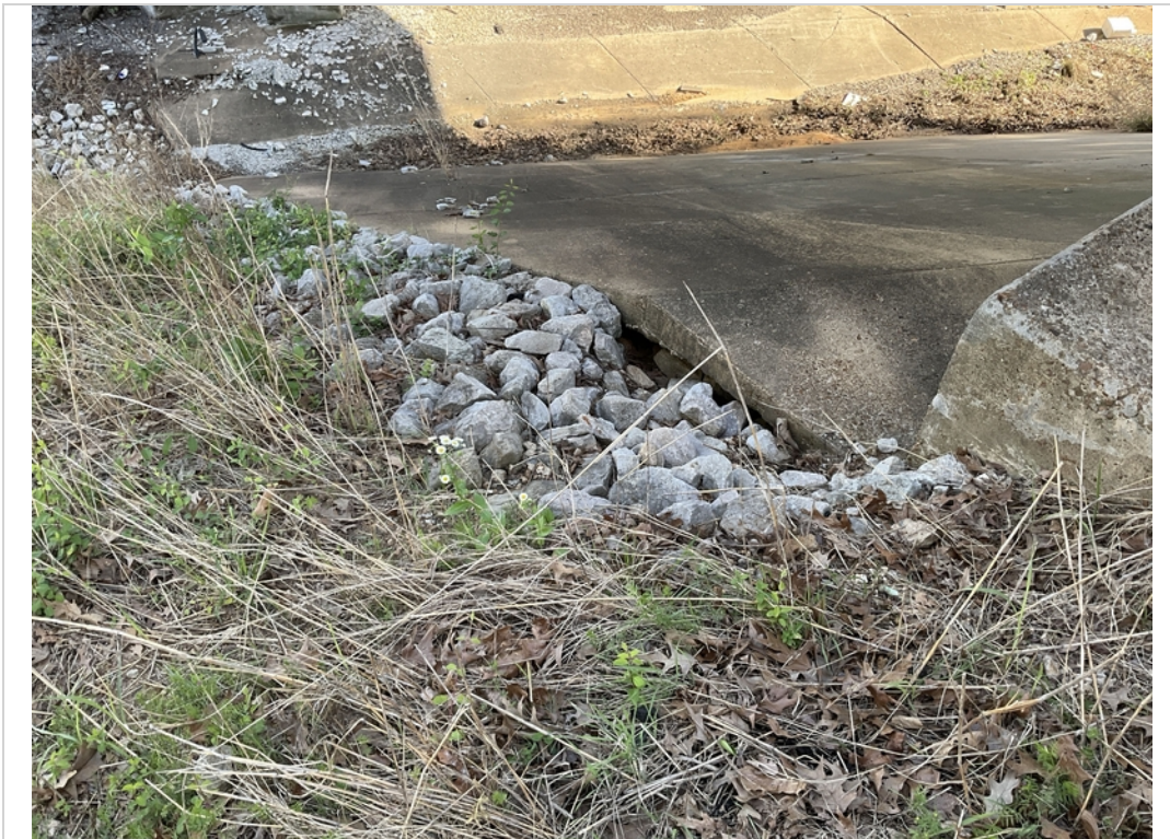
Abutment 2 right slope protection, undermining adjacent to placed rock
