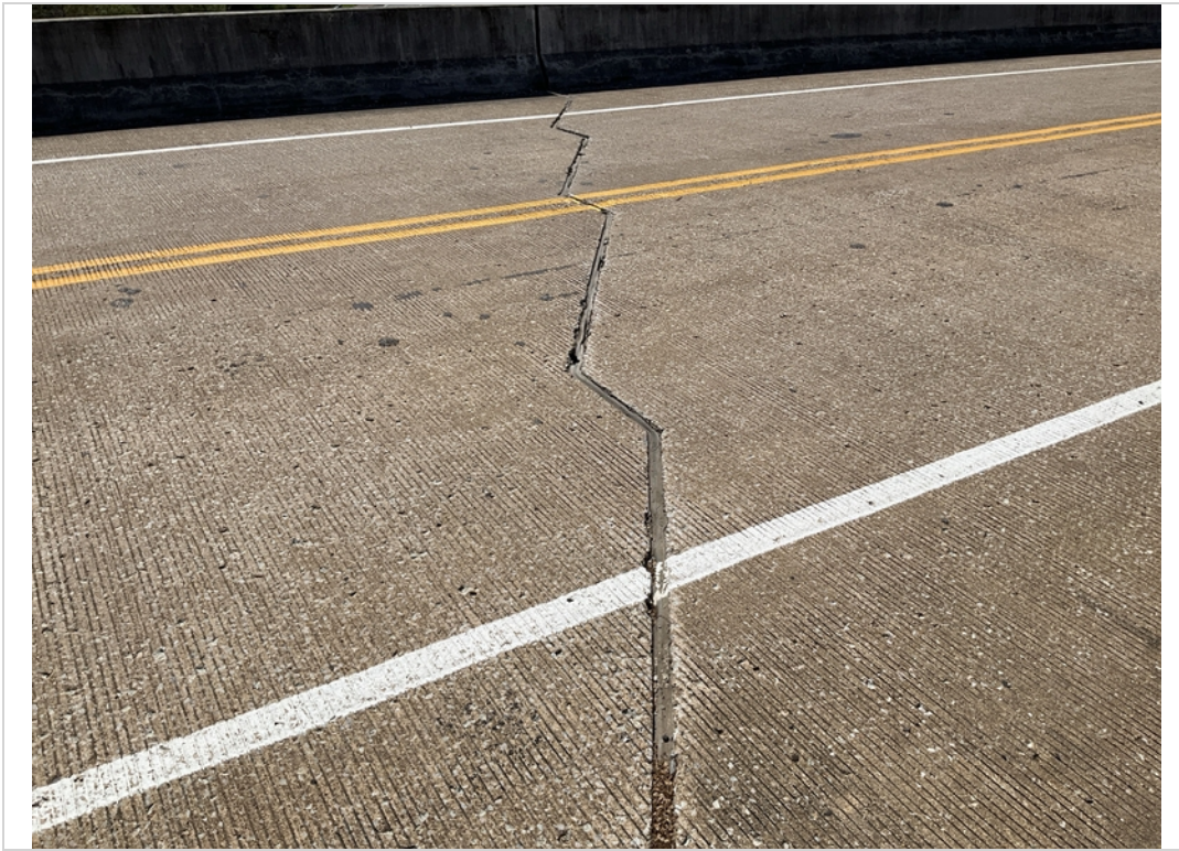
Joint over Bent 2 with failed sections of poured sealant allowing water to drain onto superstructure and substructure
