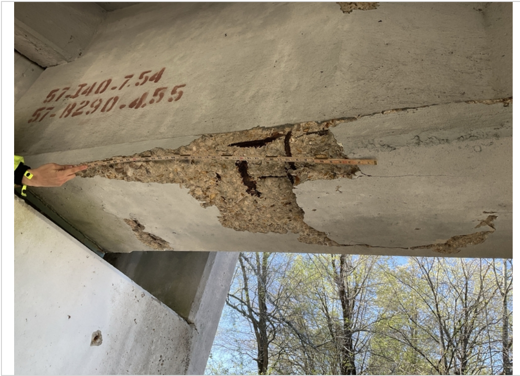
Span 1, Beam A, Abutment 1, isolated major spalling with exposing (2) P/S strands and (3) stirrups. There is longitudinal cracking along the bottom flange and delaminated areas in the beam underside and left bottom flange vertical face. Exposed P/S strand and stirrups exhibit active corrosion with minor section loss.
