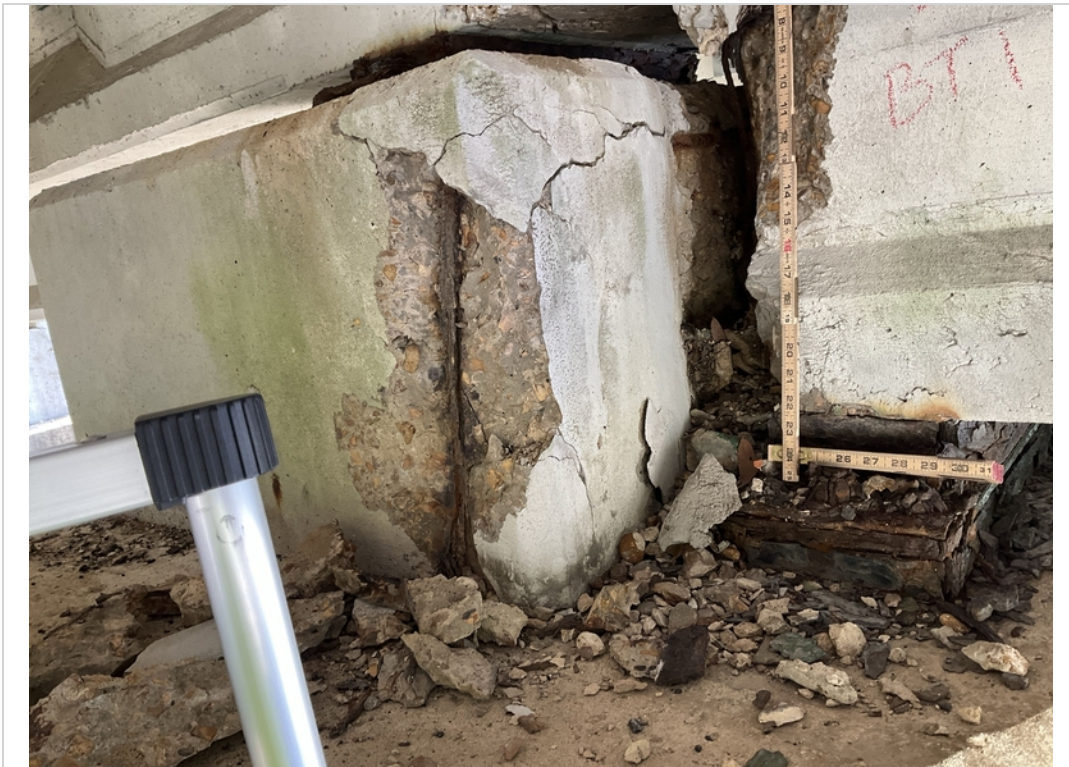
Span 1 Beam B pedestal over Bent 1, typical spall with exposed rebar. Beam end spall and heavily corroded bearing.
