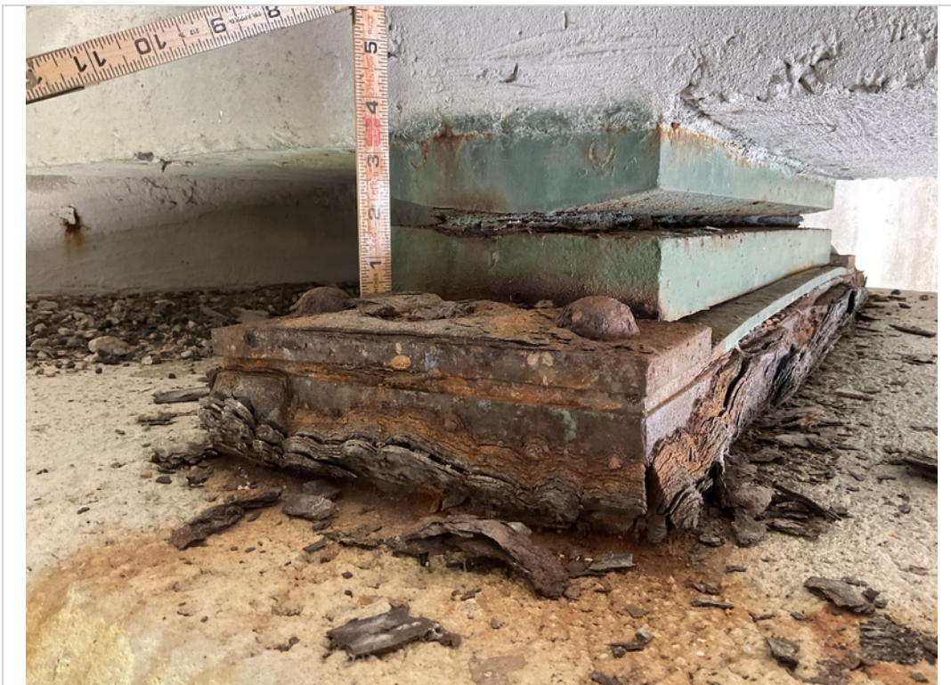
Abutment 1, Bearing D, pack rusting lifting the bearing and causing non-uniform bearing. Pack rust is 1/2" thick between sole plate and bearing plate with laminar rust along masonry plate. Missing anchor bolt at both sides.
