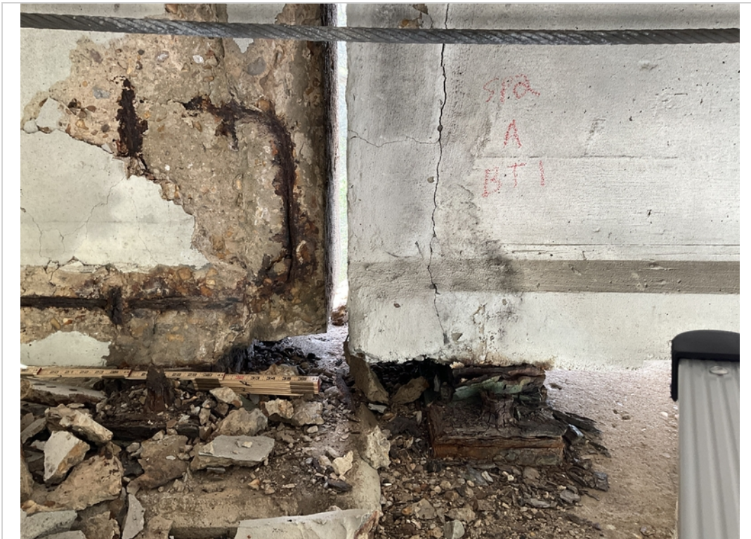
Beam A, spans 1 and 2 over bent 1, typical beam end cracking and spalling. Note corroded condition of the bearings.
