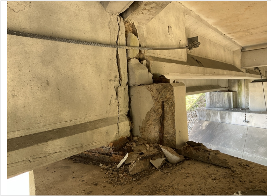
Beam D, Bent 1, spans 1 and 2, beam end delaminated areas and spalls. Pedestal spall with exposed corroded rebar.
